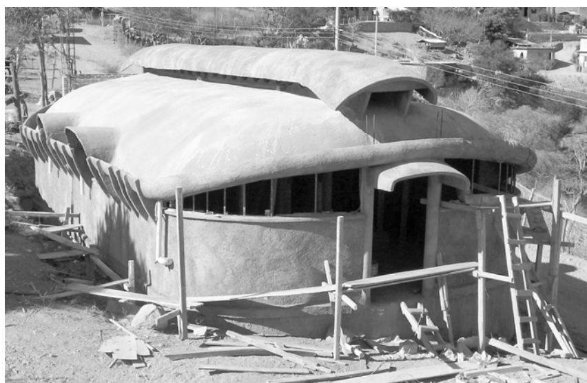
Figure 5 - Ferrocement house with water collection roofing system (courtesy Owen Waldshlaegel, New York, Intact Structures Inc.).
