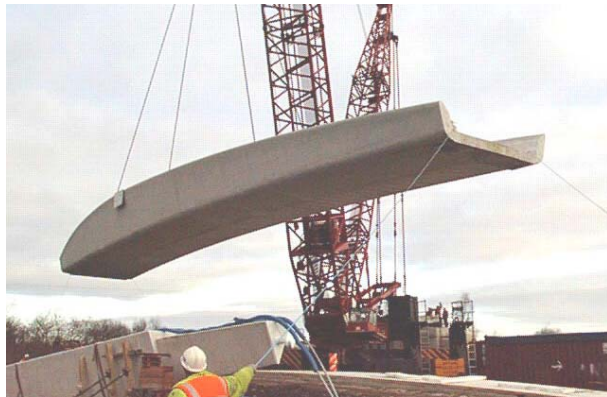
Figure 7 - Ferrocement pedestrian bridge (courtesy P. Nedwell, UMIST, U.K, and Cass and Associates, Liverpool, UK).
